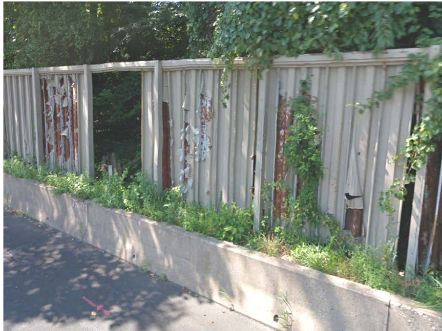
Existing Noise Barrier in Disrepair
